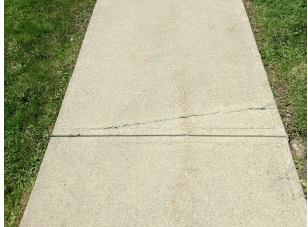
Crack at common area sidewalk
