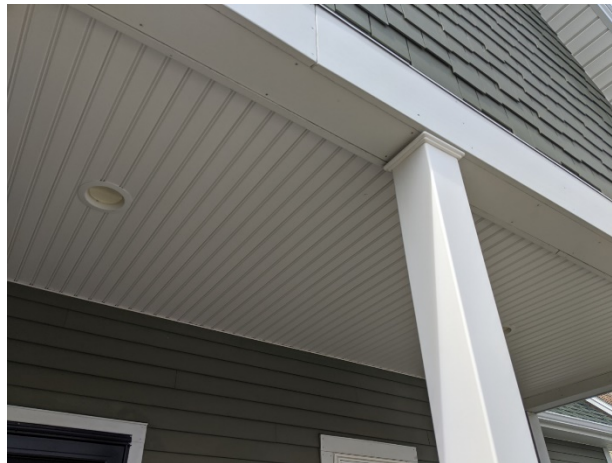
Recessed light fixture at porch soffit
