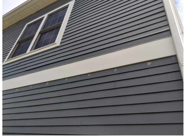
Unpainted fill at nails
