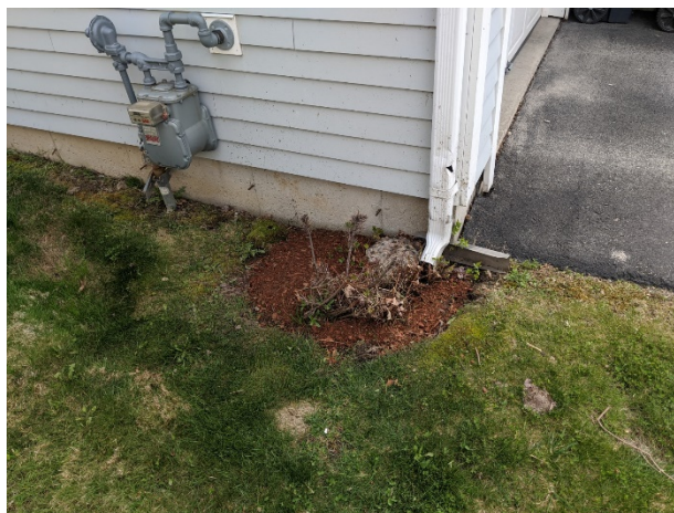
Isolated downspout damage
