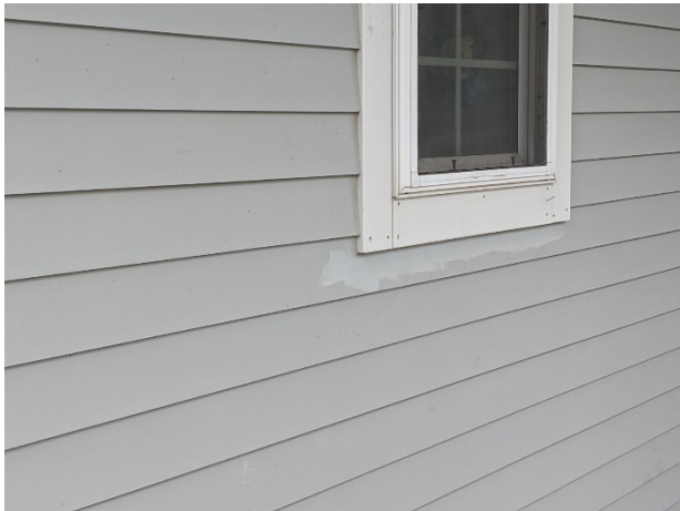
Paint finish deterioration
