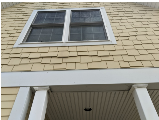
Gap between boards beneath window
