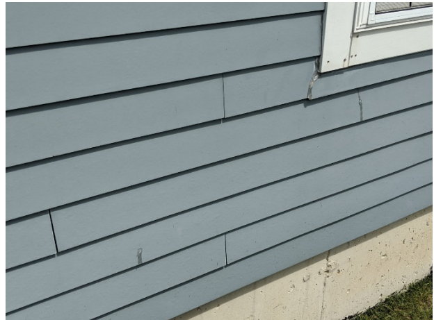
Siding damage and previous repairs
