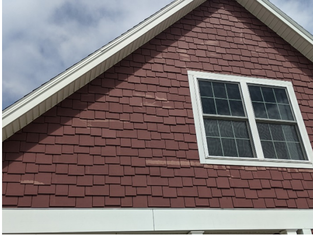
Paint finish deterioration at gable
